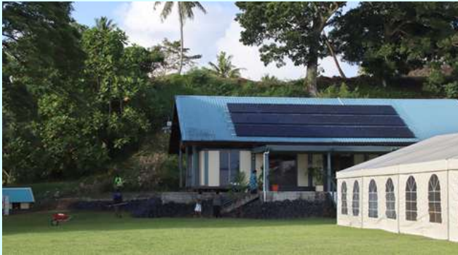
Installed solar panels in Bau Island as part of the Solarization of the Fiji State House project funded by the India-UN Development Partnership Fund.
